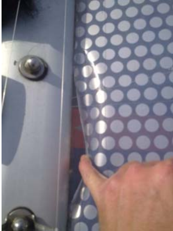
Figure 25, Failure of the weld
