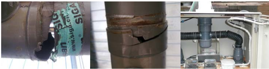
Figure 28 and 29, Clamped flexible PVC hose, broken
