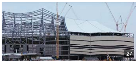
Al Bayt Stadium, Al Khor City, Qatar. Figure 24: gmp Architekten (optimization): Figure 25: Bedouin black tent. Figure 26: trussed steel structure above the reinforced concrete. Figure 27: installation of different kinds of membrane.
