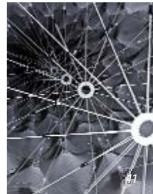
Figure 11: Tower 2, interior view: cones pulled inwards (A. Ingvarsen).
